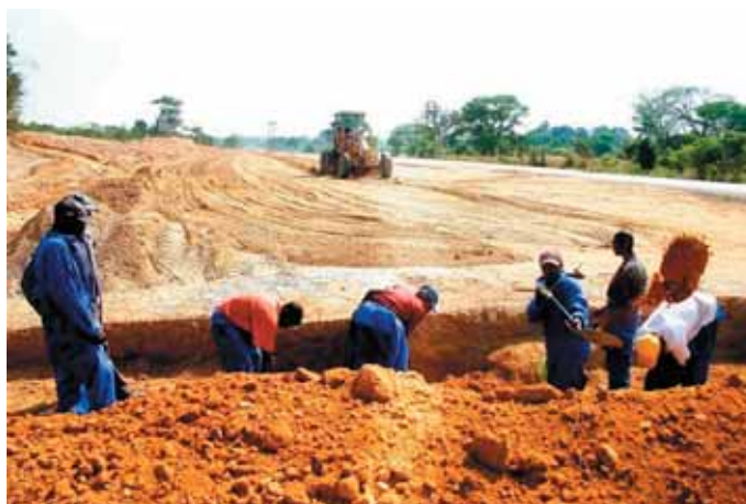
Zimbabwe is struggling to attract investors to its ambitious infrastructure development plans such as this project to dualize the Beitbridge-Harare Highway up to the Nyamapanda border post between Zimbabwe and Zambia. The project is pivotal to the Trans-Zambezi-Limpopo Development corridor, one of the key Spatial Development Initiatives envisaged to promote export-led economic recovery.
